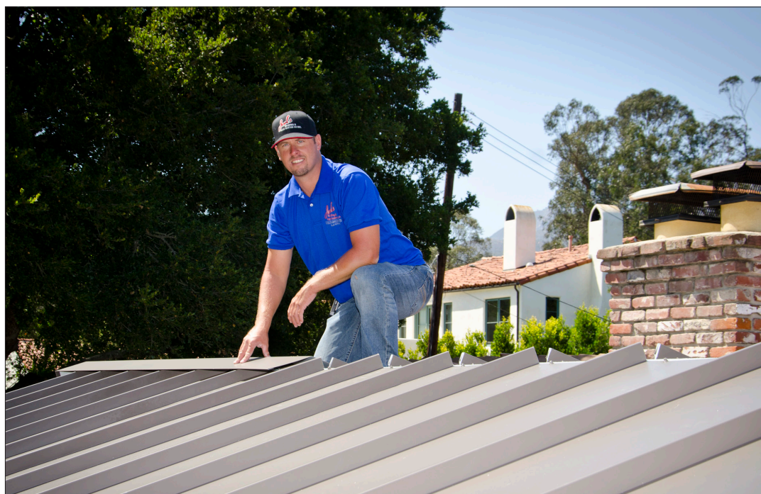
Joel's Roofing & Rain Gutter Co. owner Joel Grusinski takes to the rooftops with his fleet of bright white trucks and 10 employees.
